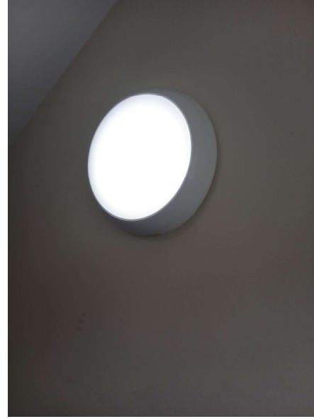
Lighting (Standard and Emergency Lights)
